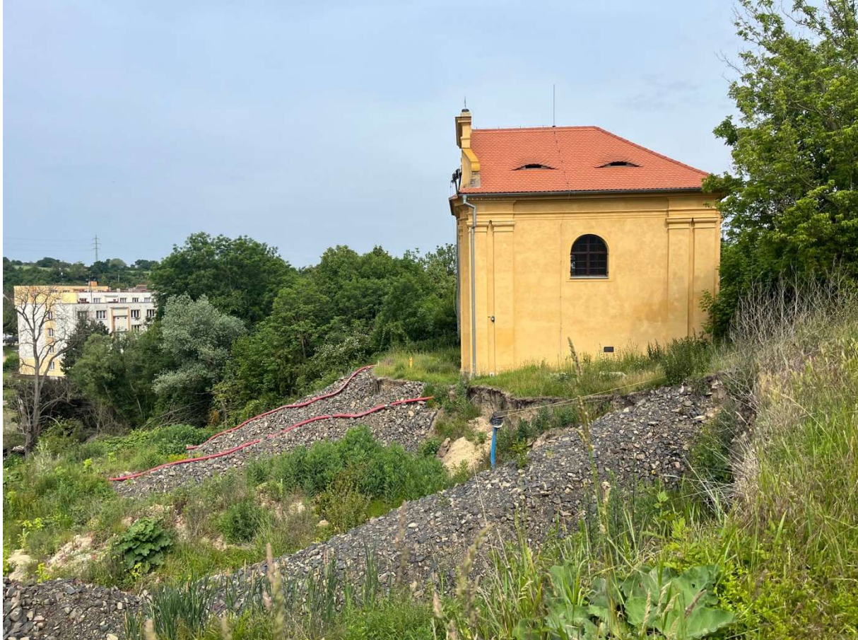
Figure 1: Landslide in Žiželice, main scarp is approximately one meter away from the Baroque chapel.
