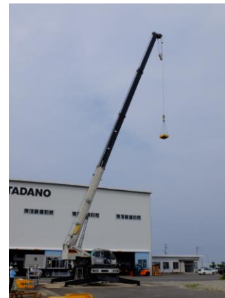
Fig.1 A crane in operation. A load is suspended to the boom and transported. A top view camera is also suspended at the top of the boom to survey the working environment.
