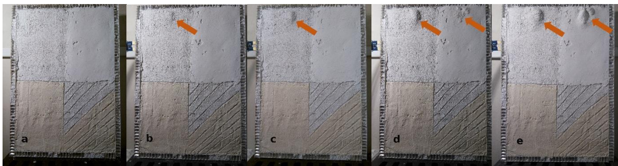
Fig. 3. Changing state of the plaster on some selected side-light pictures taken by the survey unit (a) June 2019; (b) September 2019; (c) December 2019; (d) March 2020; (e) May 2020
